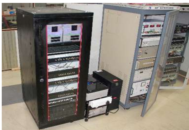
Fig. P.7.1: Compact DLLRF for Station 5 & 6 Installed in Indus-2
