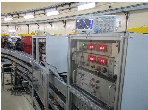
Fig. T.1.7: Commissioned power supply in Indus-2.
