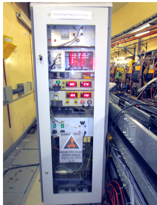
Fig. T.1.10: Commissioned vertical pinger power supply.
