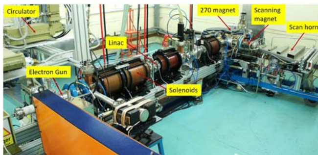
Fig. A.4.2: Linac-3 assembly under high power test.
