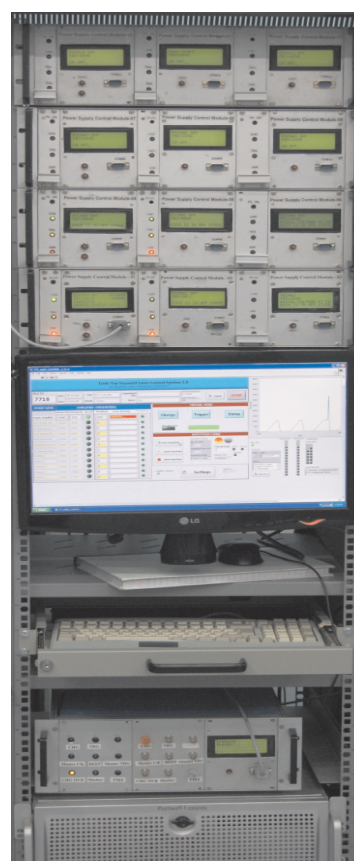
Fig. L.9.2: Photograph of the TTT control system.
