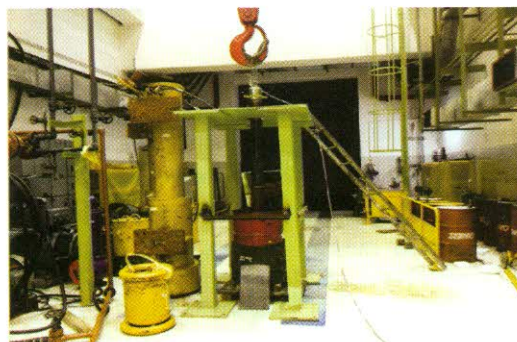
Fig. L.1.2: Underwater laser cutting set up of PT stubs at KAPS-2 site (Inset: laser cut PT stubs).
