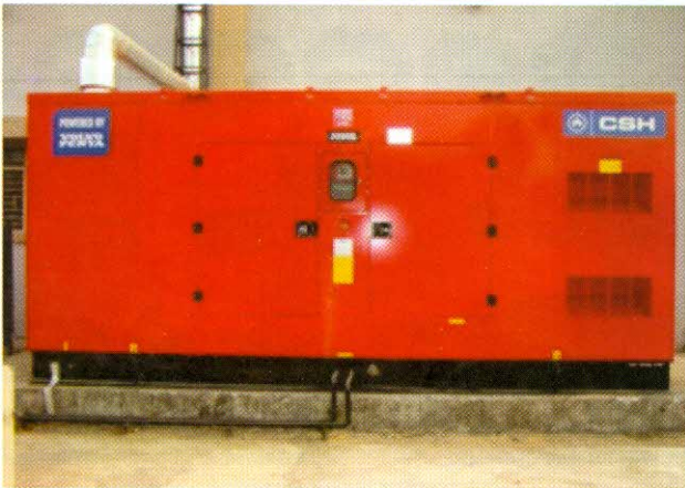
Fig. I.1.5: Front panel view of DG set at Central Complex sub-station
