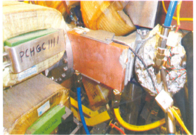
Fig. A.15.1: End plate of dipole chamber where temperature was measured
