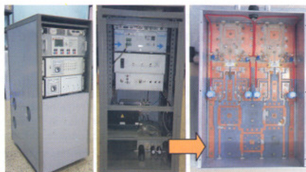
Fig A.11.1: High Power RF source for VTS. Photo from left shows the front view of complete chassis, the rear view with high power amplifier on bottom side and the inside view of the amplifier with power divider on top side and combiner on bottom side of the box.
